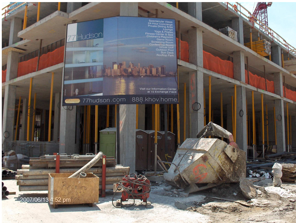
The construction site at 77 Hudson Street, a high-rise residential development in Jersey City. The complex will have two towers and 901 condominiums. Photo by Drake Rizzo and Charles Pierson, Jr. of the Department of Community Affairs.
