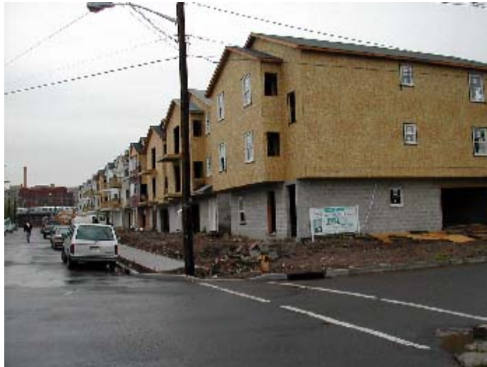
Three-family homes under construction in Newark's iron-bound district --photo by Chester Chinsky, New Jersey Department of Labor
