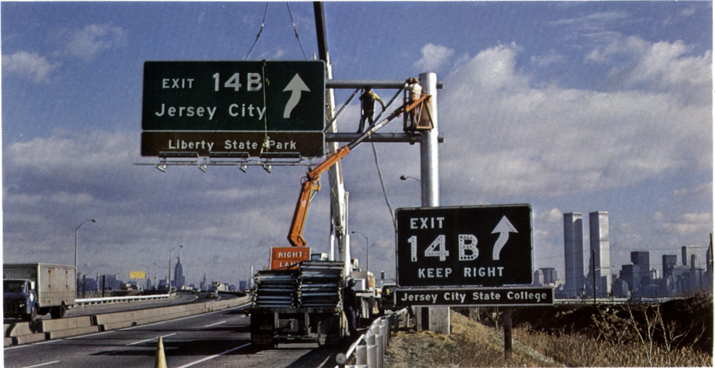
BETTER READING: New overhead signing replacing ground-mounted signs along Hudson County Extension—for easier directional guidance. Photo looking east toward N.Y. skyline and World Trade Center.
