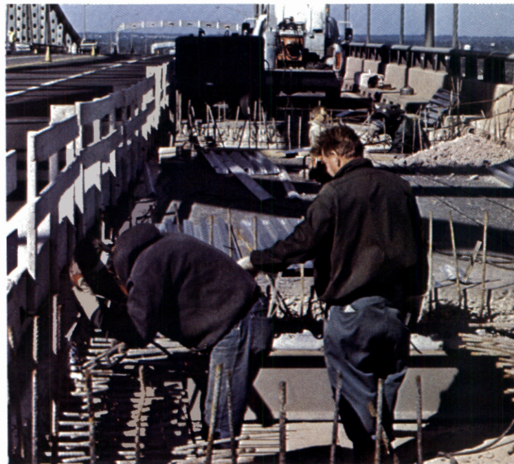
BRIDGE REPAIRS: Span linking N.J. Turnpike with Pennsylvania Turnpike undergoing repairs. Bridge over the Delaware River is jointly owned by the New Jersey and Pennsylvania Turnpikes.
