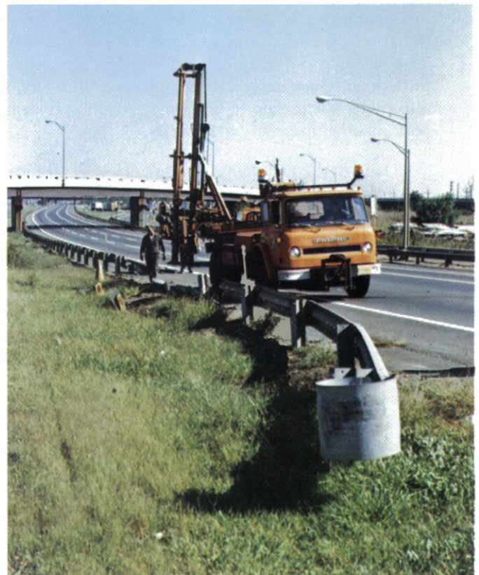
FOR EXTRA SAFETY: Repairing damaged guard rail along mainland at Elizabeth in continuing program of road safety.
