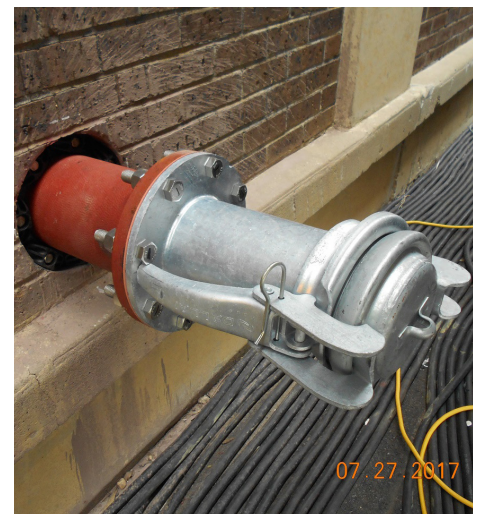
Atlantic County Utilities Authority, Trailer Mounted Portable Pumps and Permanent Sump Pump. SFY2017 Loan: $358,739
