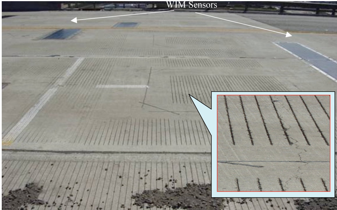
Figure 2. Crack Location and orientation in new Approach Slab at the Doremus Avenue
