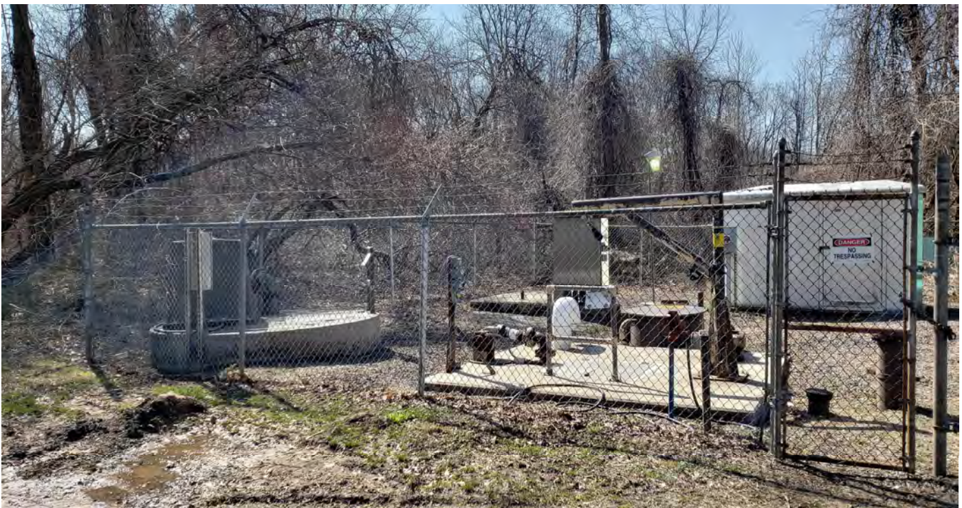
Delran Township Clay Street Pump Station. SFY2023 Water Bank Long-Term Loan: $10,288,313
