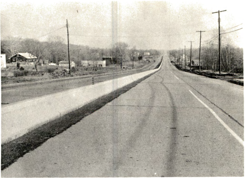
All forms being removed, the bituminous base is built up to the level of the old concrete pavement.
