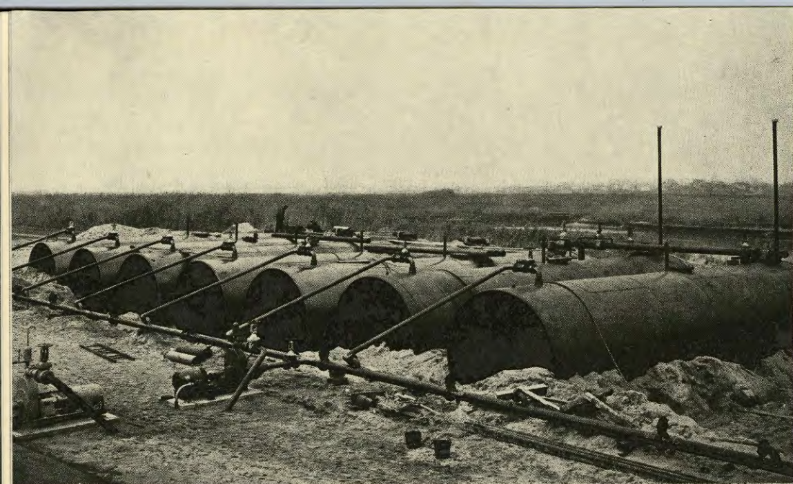
TEMPORARY TANK FARM at New York International Airport for receipt and distribution of aircraft fuel. This installation, shown under construction, is the largest temporary tank farm of its kind and comprises twenty 30,000-gallon underground tanks, located for convenient barge delivery on Bergen Basin. Construction of this $331,470 facility was begun in May and completed by the end of the year.
