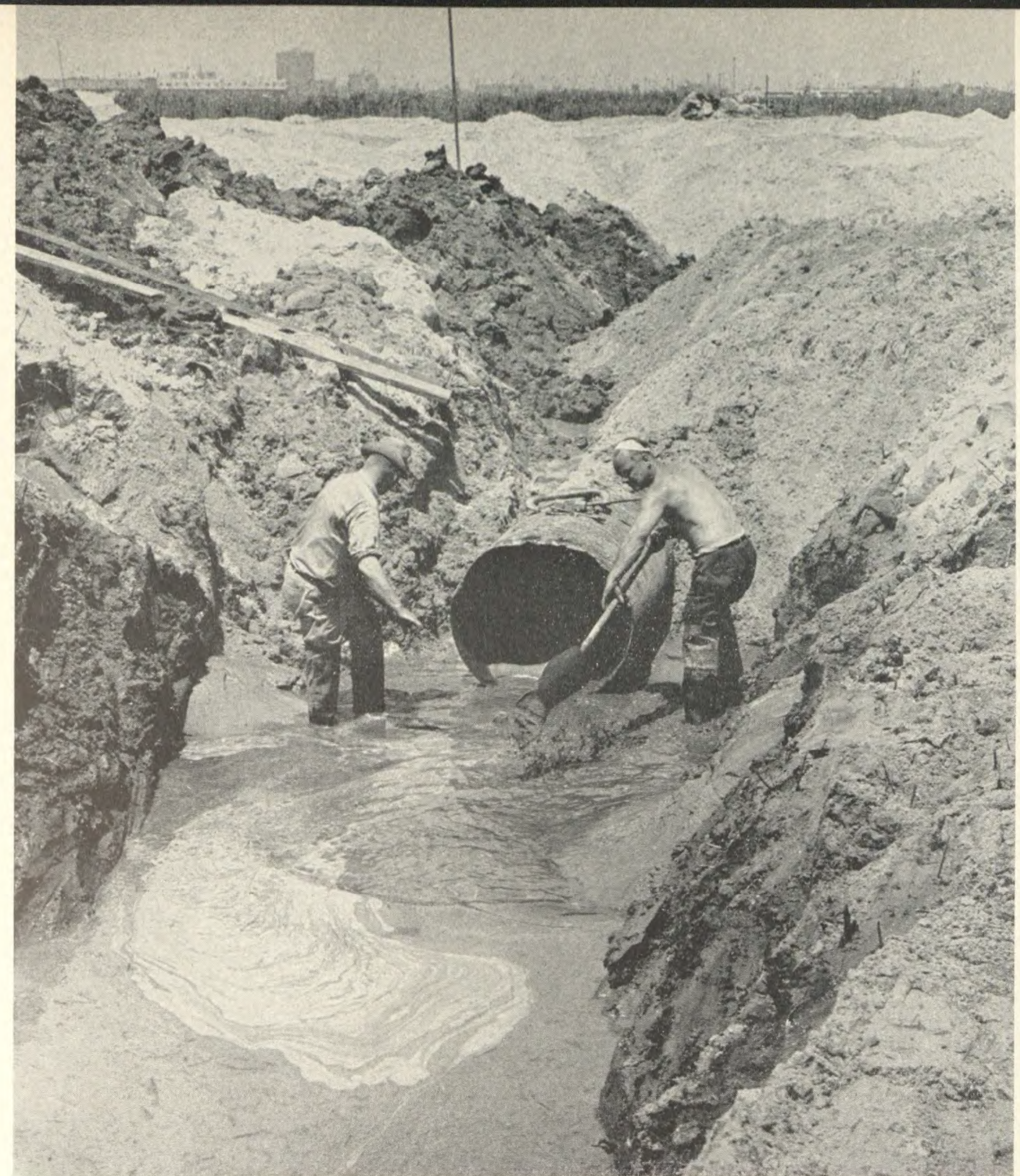
Workmen excavate ahead of this 36-inch culvert pipe, part of extensive drainage system necessary for construction of new 7,000-foot Runway A and adjoining taxiways at Newark Airport.
