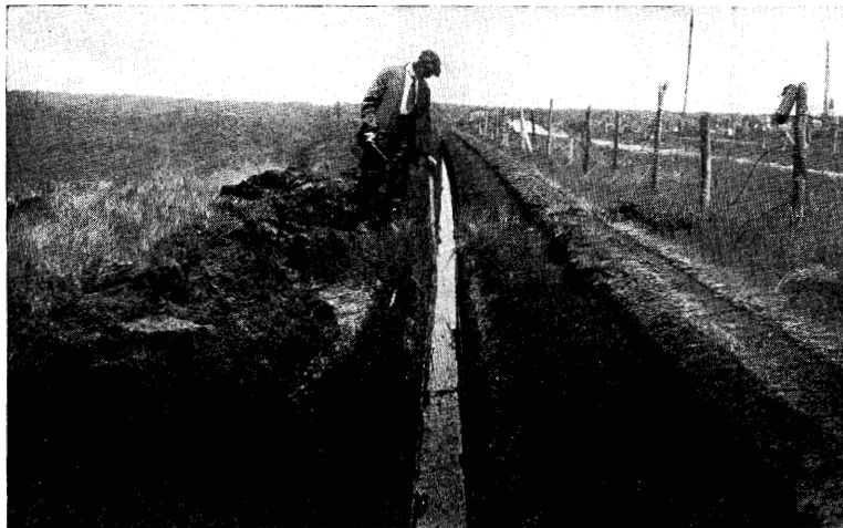
Fig. 16. A Machine-cut Ditch by Which Tidal Water is Made to Ebb and Flow and Killie Fish Given Access to Mosquito Larvæ.
