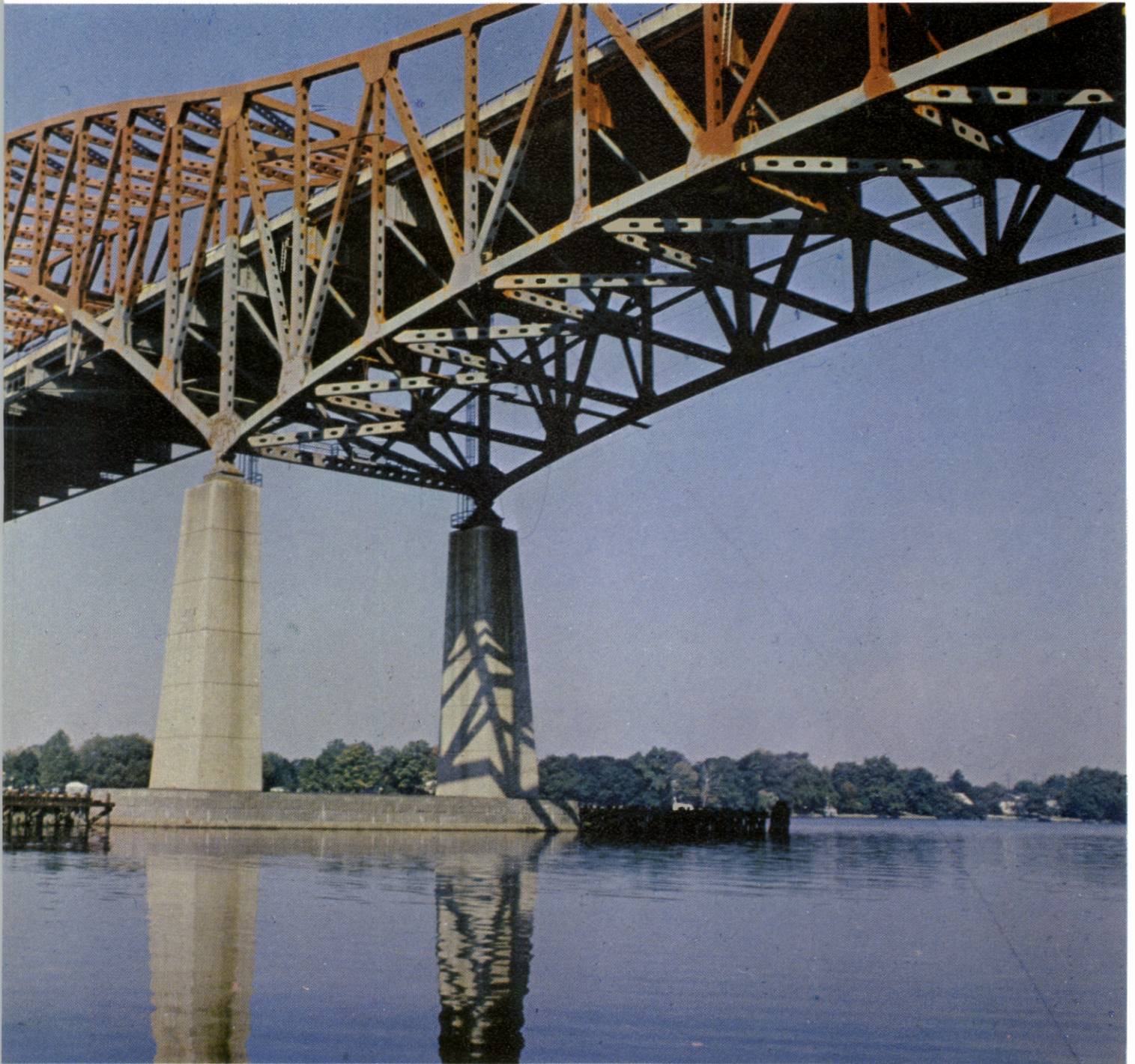
rence, connecting with Pennsylvania Turnpike. Structure maintained jointly by both turnpikes, is under extensive repair program.
