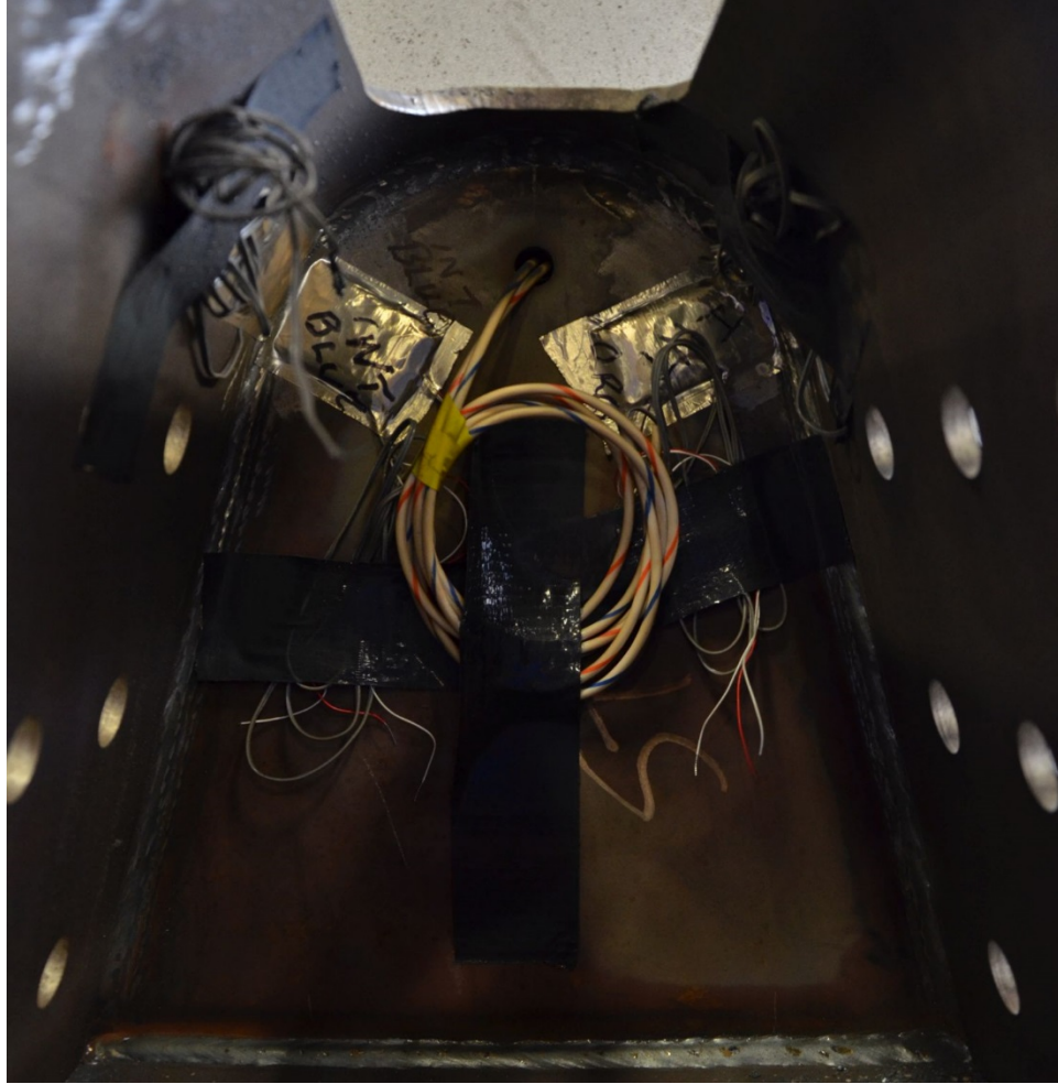
Figure 369. Installation of gauges on rib wall and sealing plate at rib-to-sealing plate connection at HIS facility
