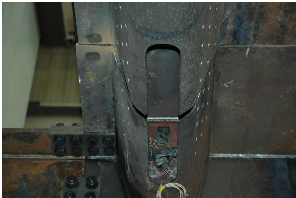
Figure 351. Lack of alignment of the ribs
