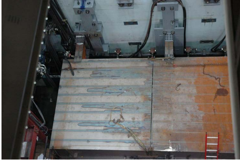
Figure 346. Heat marks on the deck after heat treatment
