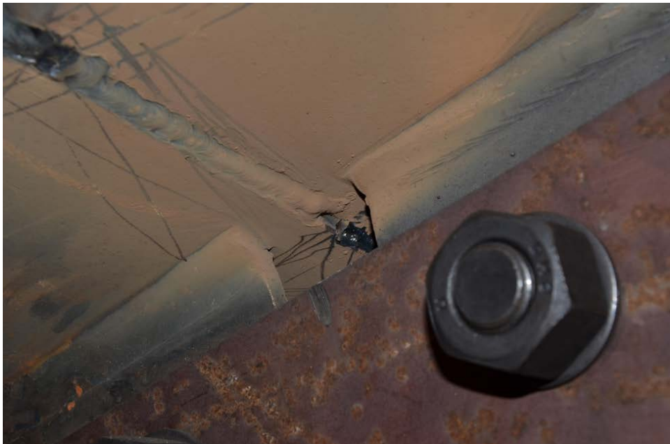
Figure 359. Lack of access over the rib wall for re-welding
