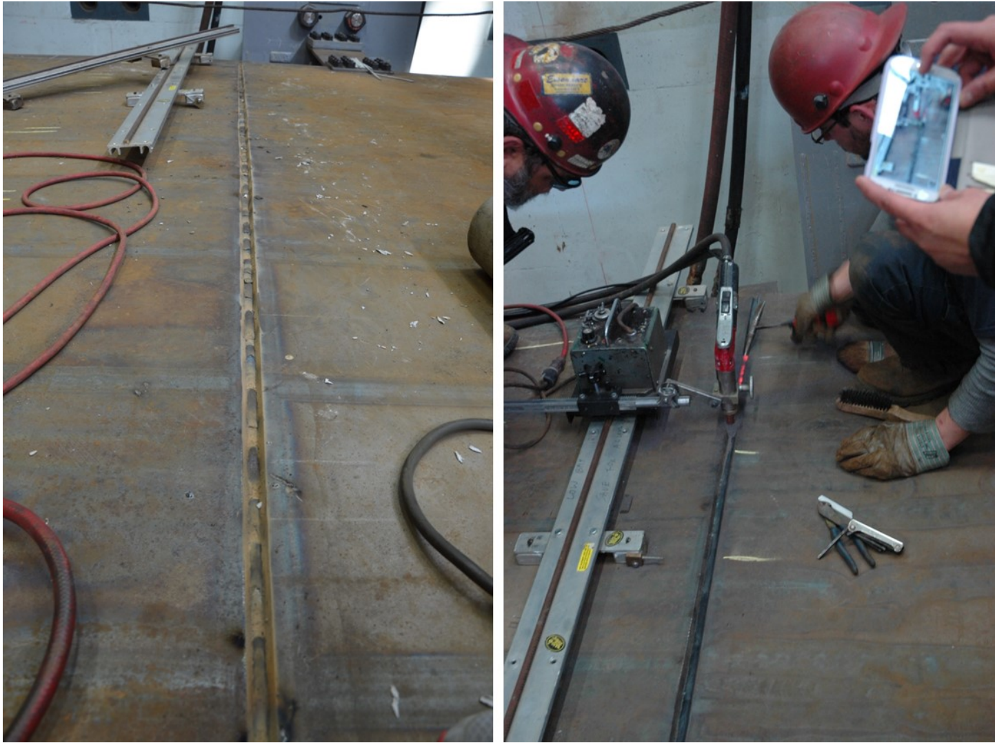
Figure 353. Root pass and fill pass for the CJP weld at the transverse deck splice at deck plate
