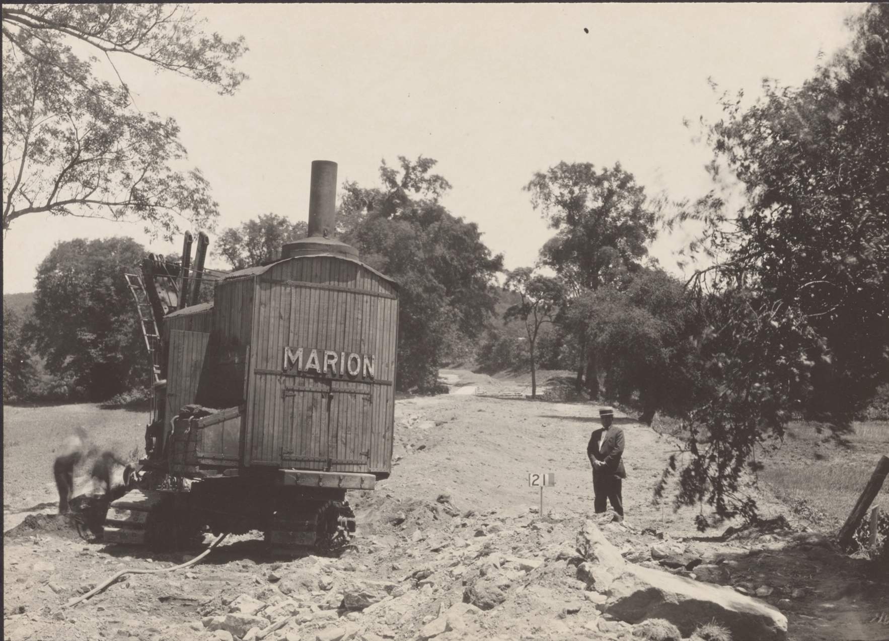
NO. 21 VIEW SHOWING FILL ON SITE OF MORRIS CANAL SOUTH OF PEER'S LOCK AT DENVILLE JUNE 11, 1925
