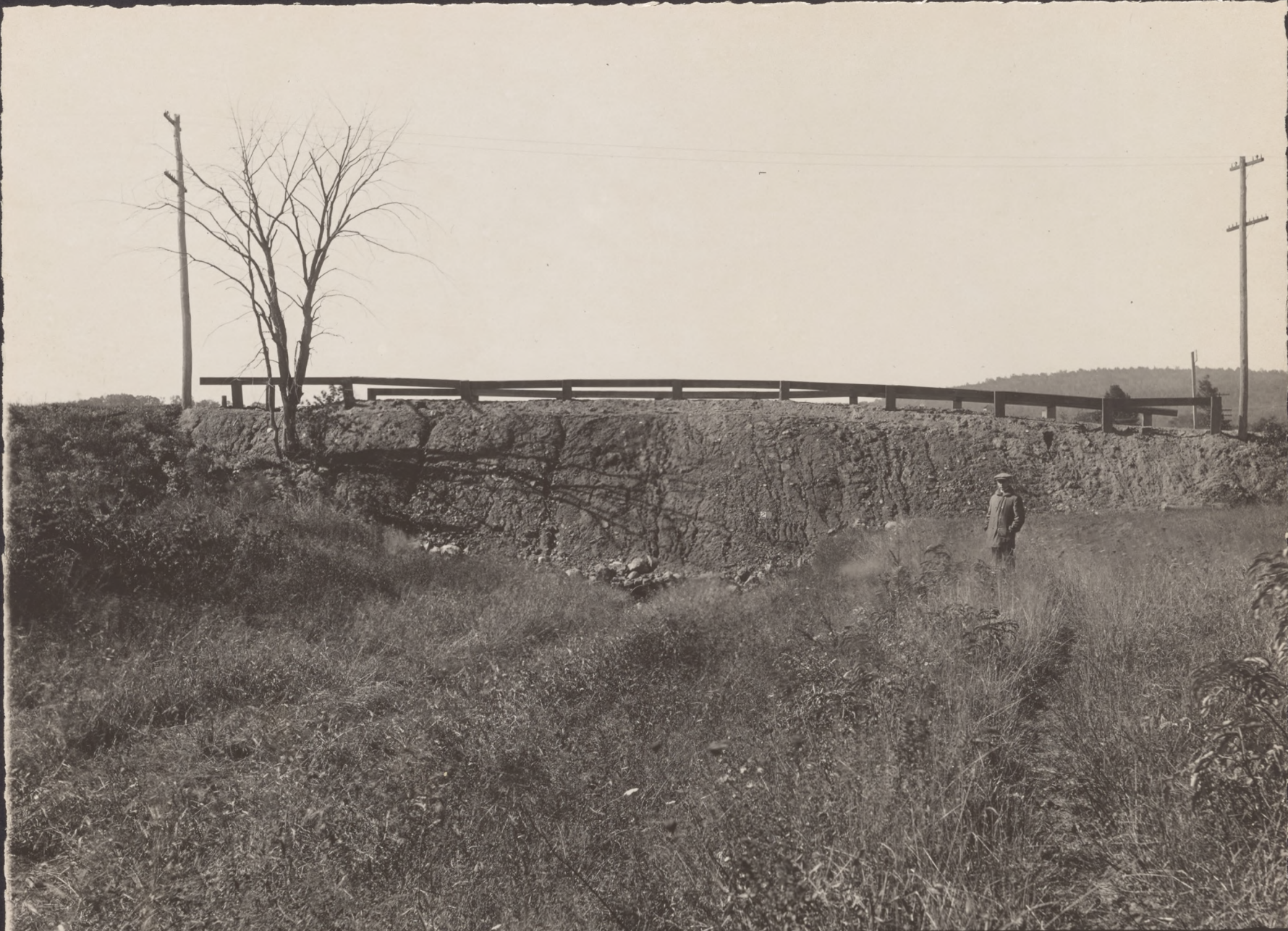
N o 2 FILL IN MORRIS CANAL AT SITE OF "CHANGE BRIDGE" IN LOWER MONTVILLE VIEW LOOKING NORTH
