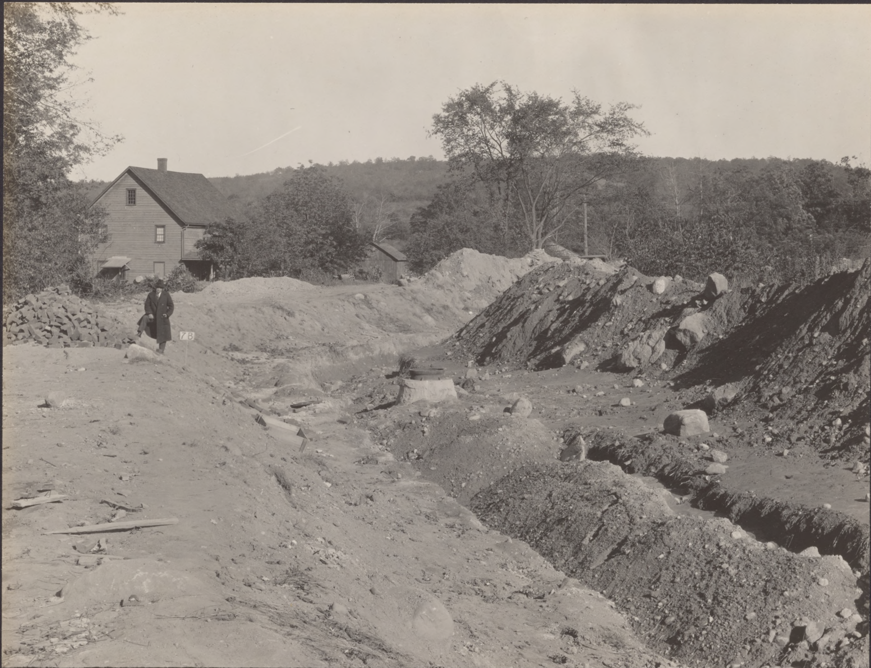
NO 7B SEWER CONSTRUCTION IN BED OF MORRIS CANAL 300 FEET WEST OF BRIDGE #84 ABOVE BOONTON VIEW LOOKING EAST
