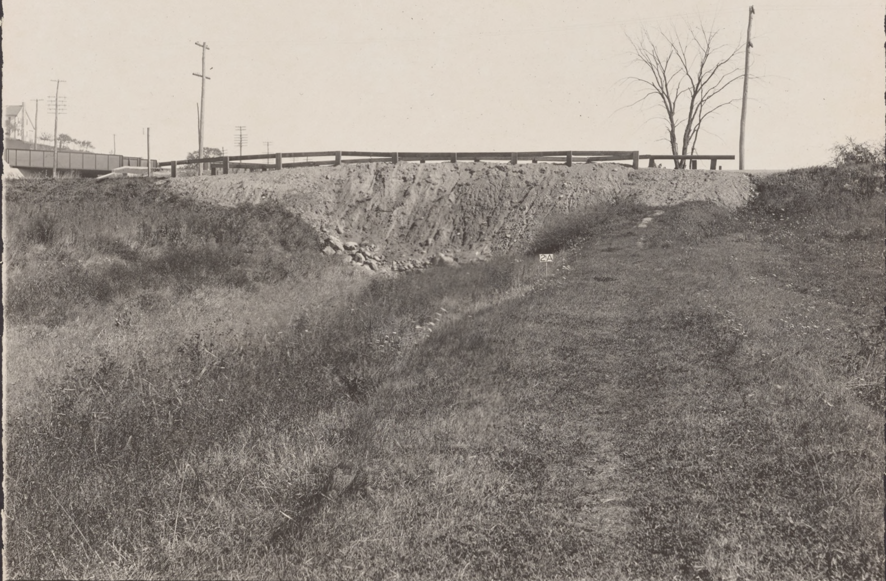
NO 2A FILL IN MORRIS CANAL AT SITE OF "CHANGE BRIDGE" IN LOWER MONTVILLE VIEW LOOKING SOUTH
