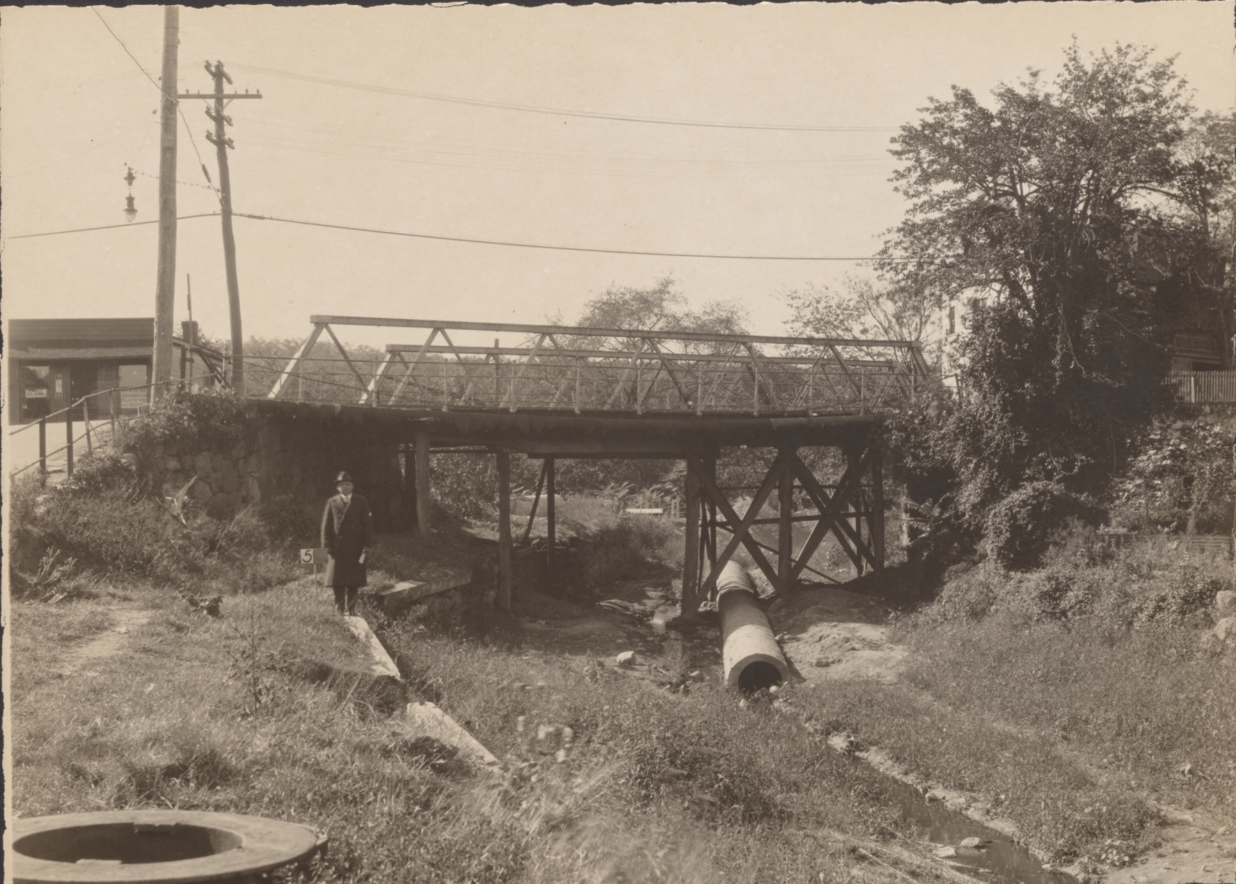
NO 5 SITE OF PROPOSED FILL - MORRIS CANAL - MAIN ST BRIDGE AT BOONTON VIEW LOOKING NORTH WEST OCT 9, 1924.
