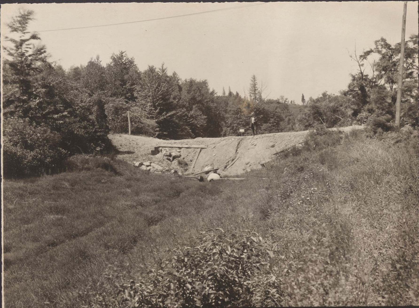
NO. 25 SITE OF ROAD BRIDGE CROSSING MORRIS CANAL AT TOWACO LOOKING WEST
