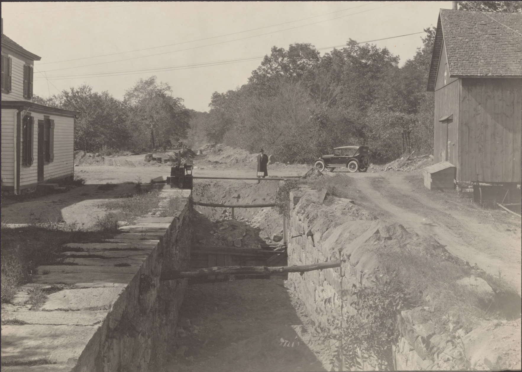
No 9 FILL IN MORRIS CANAL - MAIN ROAD CROSSING AT PEER'S LOCK NEAR DENVERVILLE VIEW LOOKING NORTH OCT. 10, 1924
