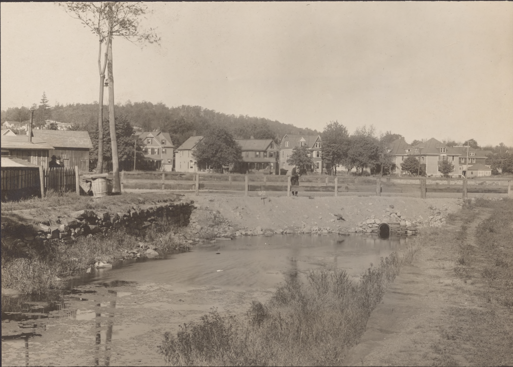
N o 10A FILL IN MORRIS CANAL AT EAST CLINTON ST. - DOVER VIEW LOOKING EAST OCT. 10, 1924
