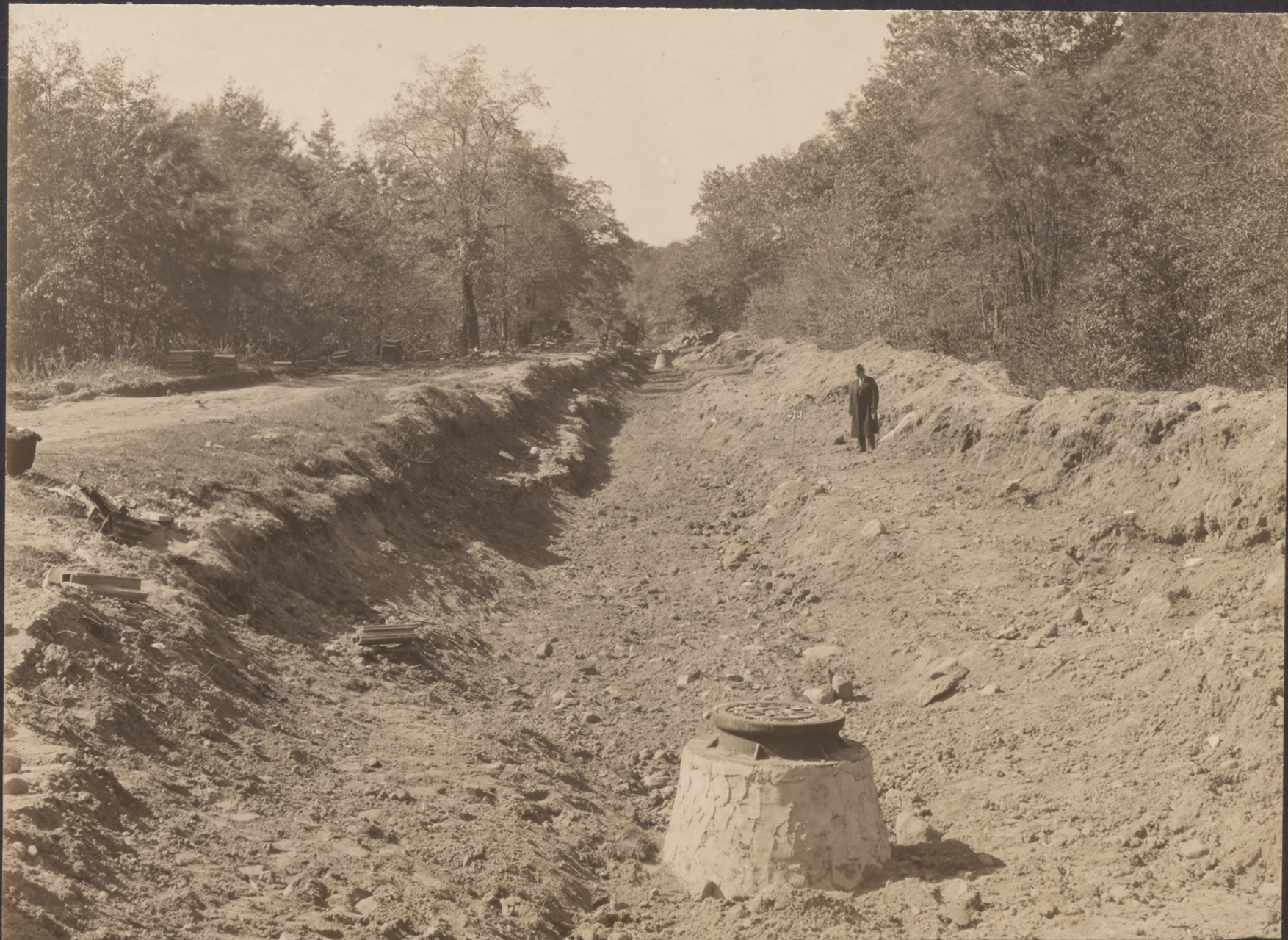
NO 98 SEWER CONSTRUCTION IN MORRIS CANAL NORTH FROM PEER'S LOCK NEAR DENVER OCT. 10, 1924
