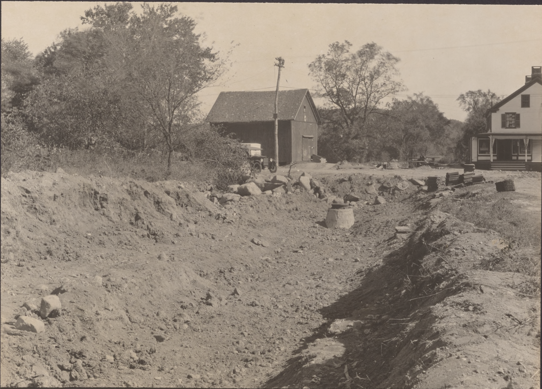
NO 9A FILL & SEWER CONSTRUCTION IN MORRIS CANAL-MAIN ROAD CROSSING AT PEER'S LOCK NEAR DENVILLE VIEW LOOKING SOUTH
