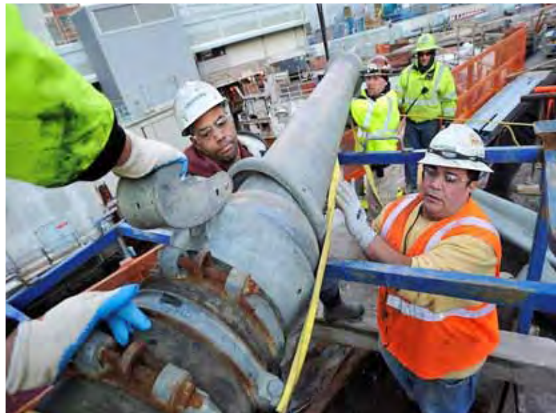
The Port Authority established a 15 percent goal for qualified Disadvantaged Business Enterprises. Projects include the installation of flood barriers, drainage systems, and structural protection for station infrastructure.
