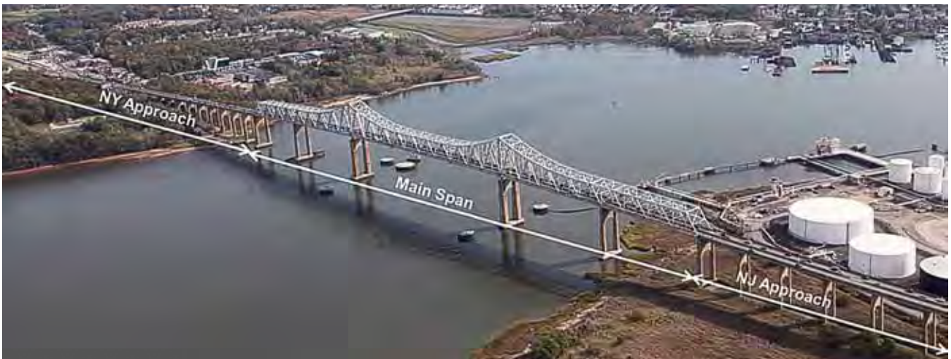
Construction crews worked overnight and on weekends to pave the Outerbridge Crossing in 2013.
