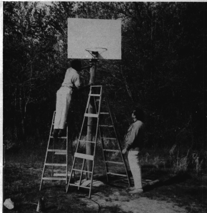
NEW NETS — Charles Palmer (left), 17, of Whitesboro, helps construct a temporary basketball court, the first to be located in this community. The court is now used by local youngsters who previously had to travel six miles to play the sport. Looking on is Samuel Kriegman of the Community Affairs Department, which acquired the nets and the materials.
