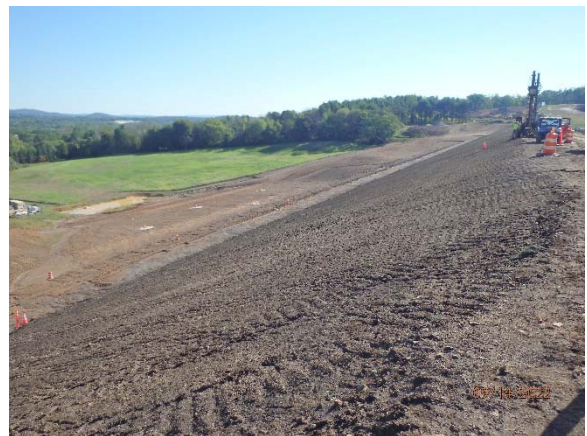
Major earthwork was completed at the North Dam in the summer of 2022. Restoration work, including placement of topsoil, and installing permanent instrumentation is ongoing.
