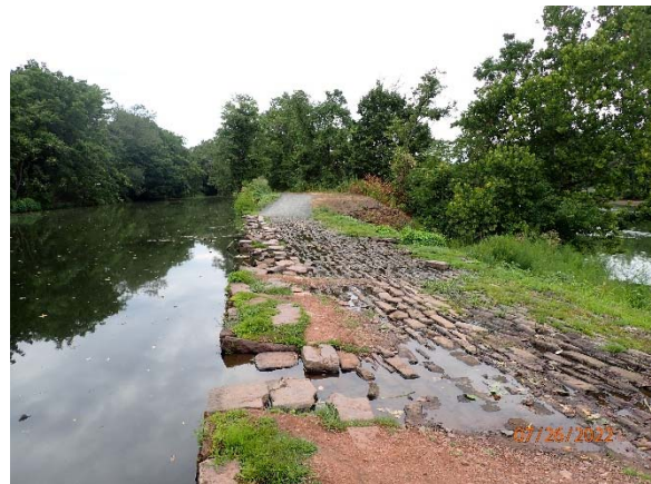
Crest of the Landing Lane Spillway. In 2021, flooding from remnants of Hurricane Ida washed away most of the towpath screenings which had previously covered the crest.
