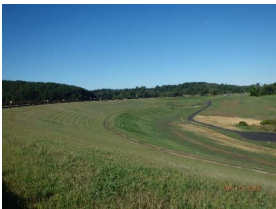
Ongoing and recent restoration work at the Dike includes establishing grass, instrumentation wiring, and security fence installation.
