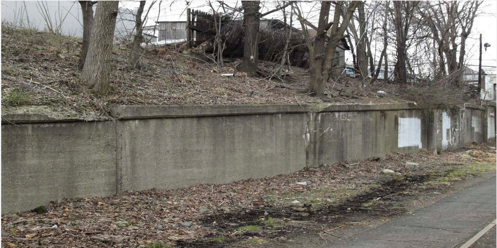
Deteriorated infrastructure surrounding the station.
