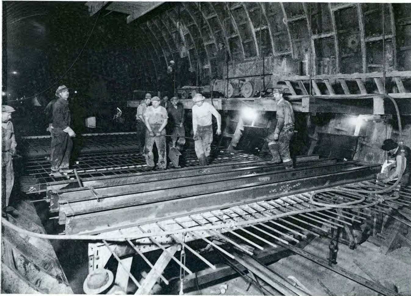
Midtown Hudson Tunnel—General View of Roadway Construction, New York, Placing of Beams and Reinforcing, Looking East October 24, 1935
