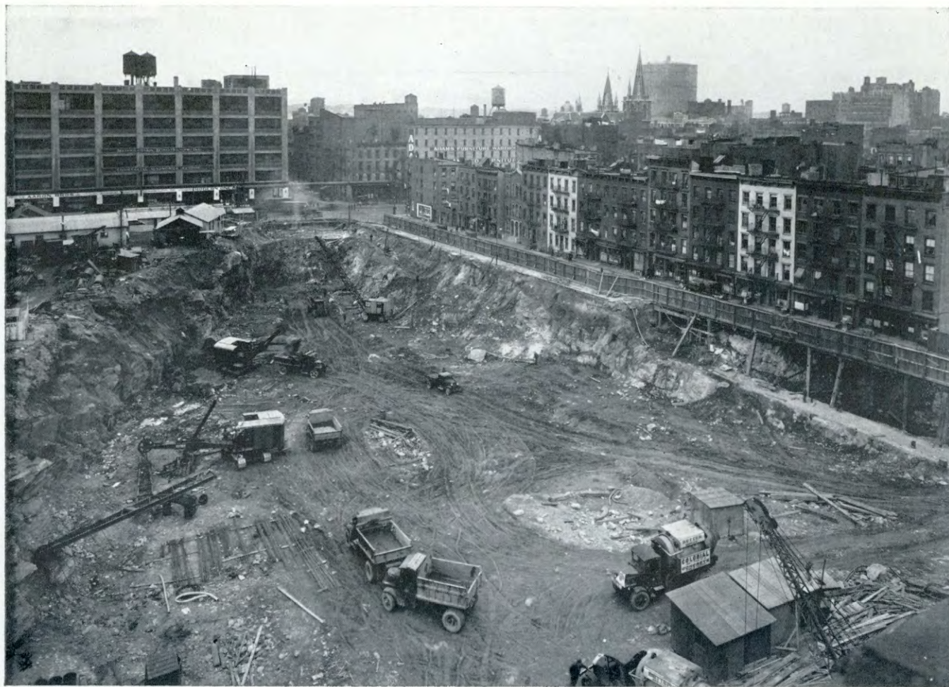
Midtown Hudson Tunnel—New York Approach. Excavation for Plaza and Portal Area, Looking Northwest from West 38th St. December 3, 1935
