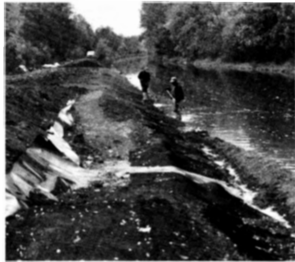
Additional seepage along Edgewood Avenue required extension of the liner in the Canal embankment.
