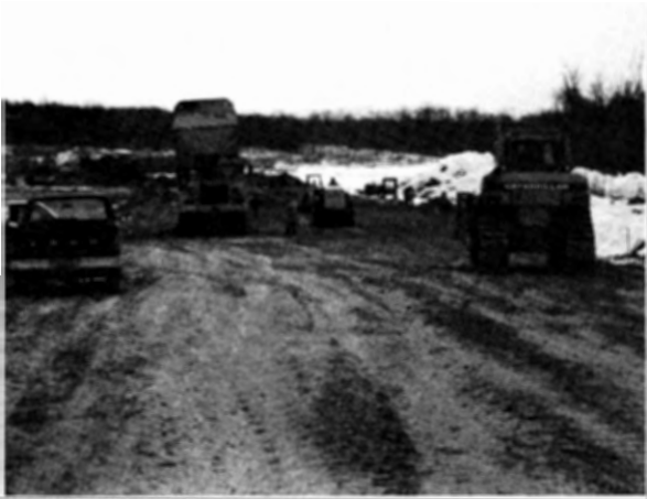
Installation of the temporary earthen embankment cofferdam to control flood flows in Timber Swamp Brook upstream of the site of the Manasquan Reservoir Dam.
