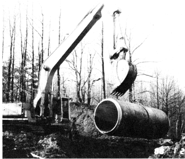
Installation of the 66" pipeline between the intake facility and the Manasquan Reservoir site is proceeding ahead of schedule.
