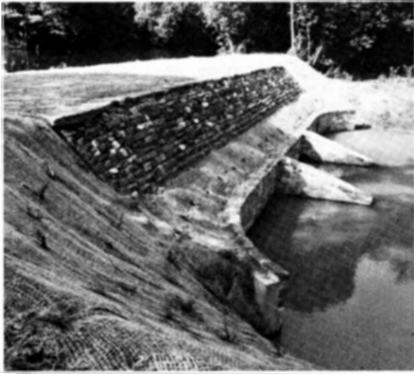
The rehabilitation of Ten Mile and Six Mile culverts in Franklin Township was completed.
