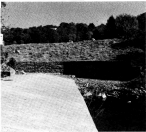
Completed Gabion wall repair of the Canal embankment washout at the wing dam in the Delaware River near Lambertville.
