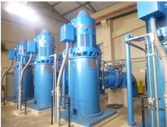
Variable speed motors on reservoir fill pumps
