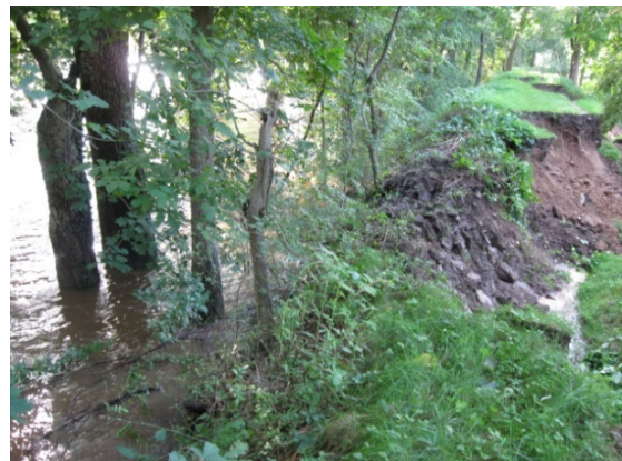
D&R Canal embankment in Stockton Borough in 2011.
