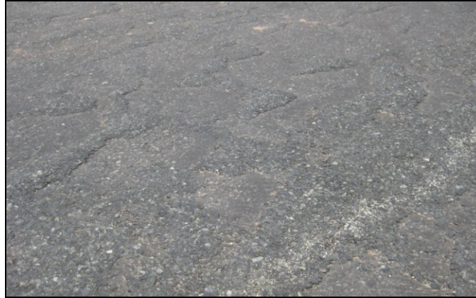
Figure 46. Road Surface. The surface of the road was noted to be rough and uneven.
