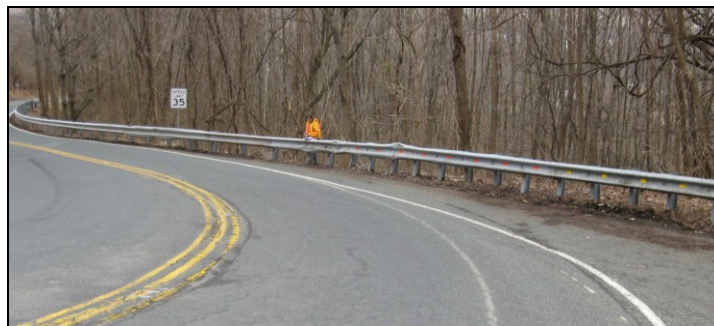
Figure 45. Damage to guardrail. There is notable damage to the rail and the posts in multiple areas.
