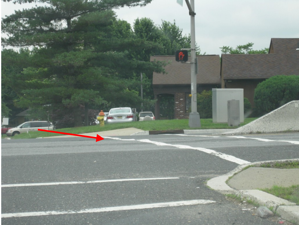
Figure 53. Surface roughness at intersection of Route 35 and Miller Avenue in Hazlet Township, Monmouth County
