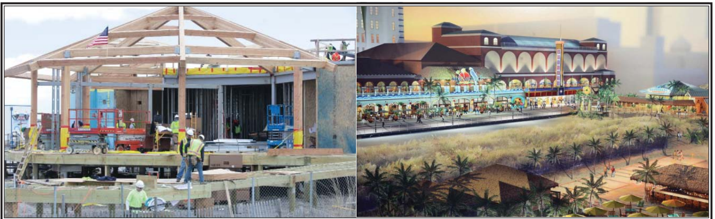
Construction has commenced for the new Landshark Bar and Grill, which will soon become part of the new “Margaritaville” complex of Resorts Casino Hotel.
