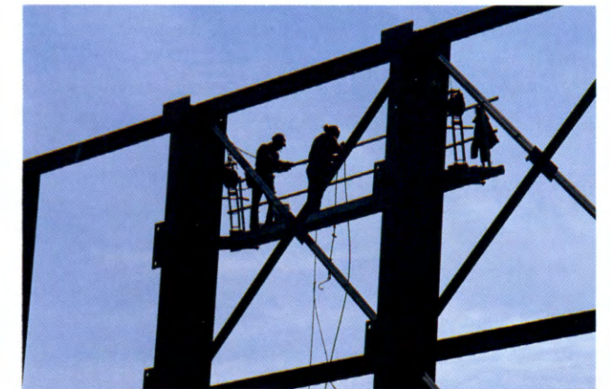
Construction of a radio frequency interference shield wall and infield at Teleport, a satellite communications center in Staten Island.
