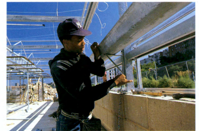
A new Business-Technology Center under construction at Bathgate Industrial Park in the South Bronx.
