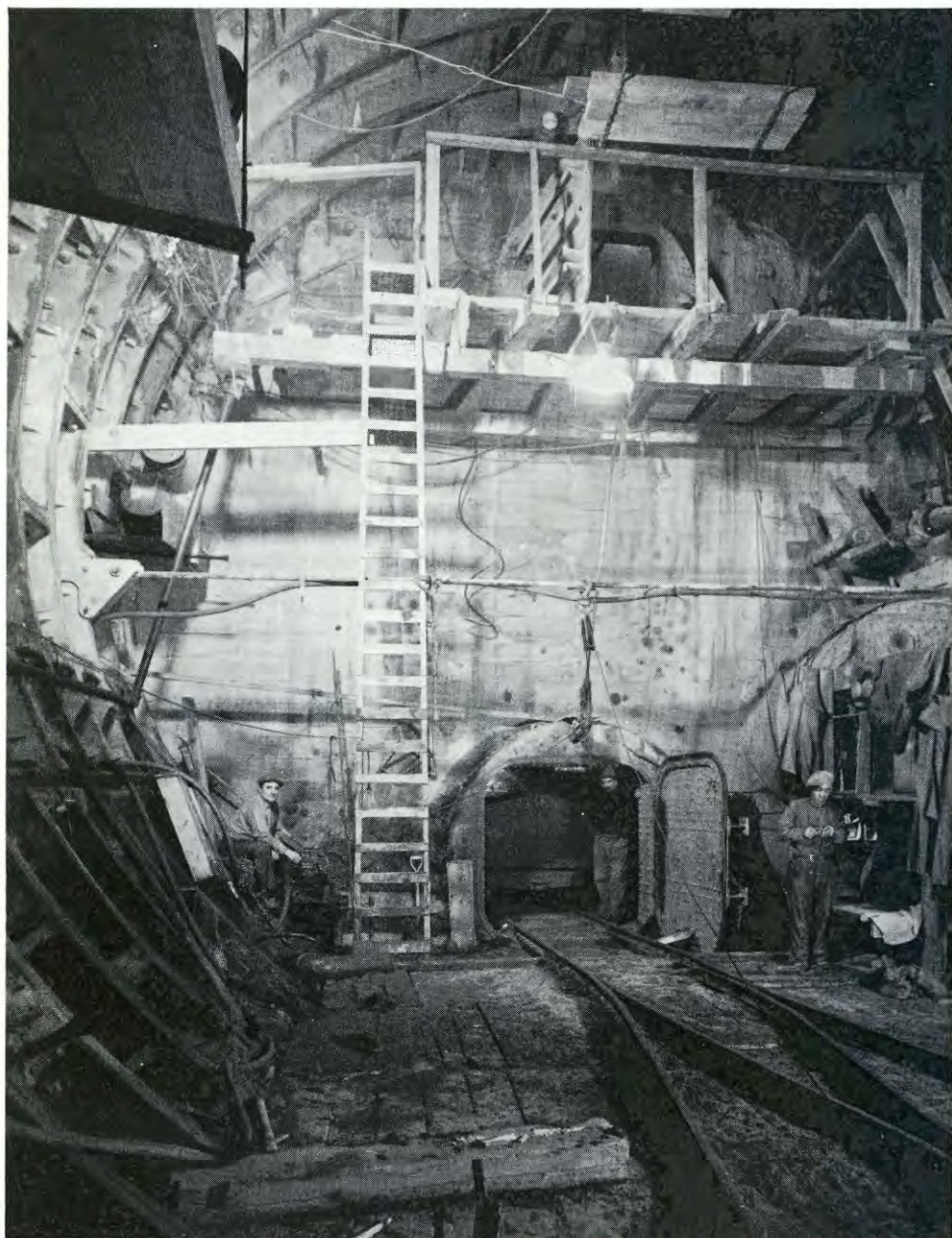
Midtown Hudson Tunnel—Concrete Bulkhead at West End of Compressed Air Chamber— Weehawken, N. J. January 10, 1935
