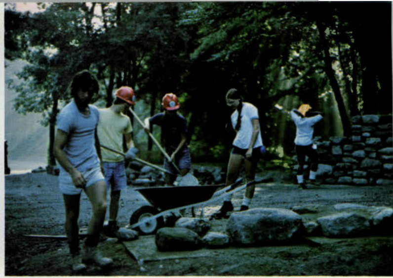
Workleader Dan La Poma, River Edge, leads his work group in constructing new stone pillars at the entrance to Stoney Lake.
