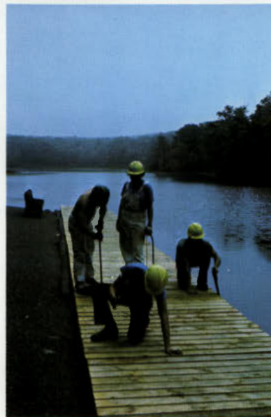
YCC'ers put the finishing touches on new boat dock at Stoney Lake.
