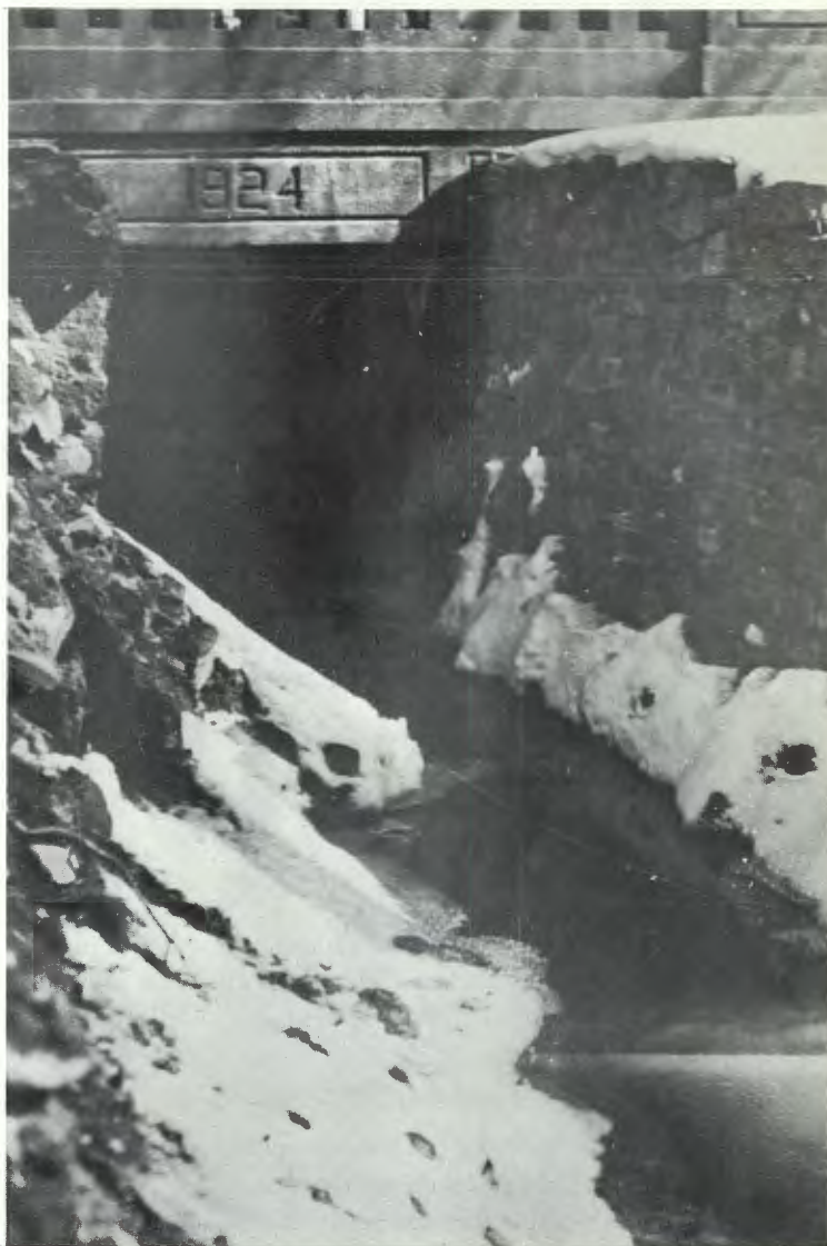
An encroachment violation occurs when the smooth flow of water is illegally impeded. Such a violation is pictured here.
