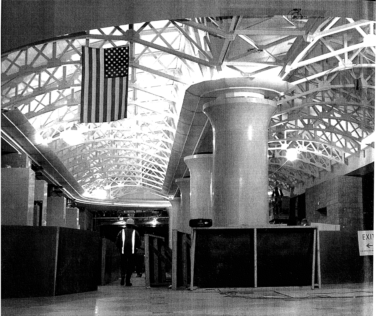
NJ TRANSIT 7th Avenue Concourse, Penn Station New York, under construction in 2001
