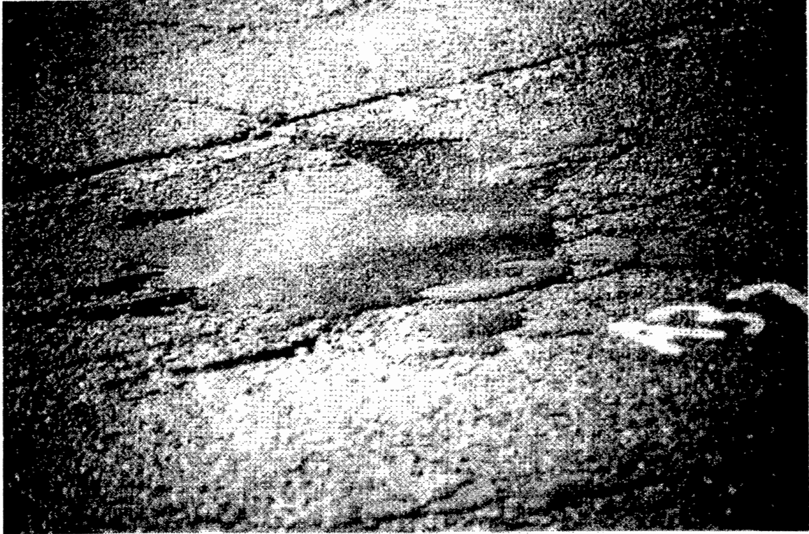
Figure 3. Edge Disintegration Distress (3)
