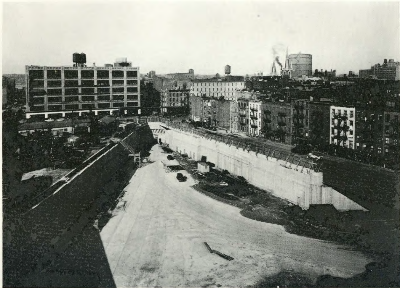
Midtown Hudson Tunnel—New York Open Cut Looking Toward South Tunnel Portal. (10th Ave. and 39th St.)
