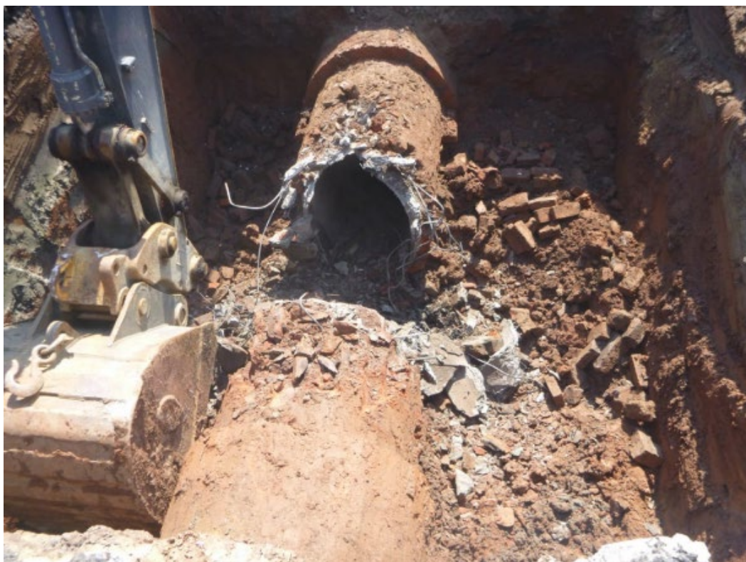
Figure 90. Wire mesh used in the gunite rehabilitation of the Trumbull Street brick sewer. Source: Ilene Grossman-Bailey and Laura D. Cushman, Trumbull Street Flood Control Project, Trumbull Street, East Sixth, Street and Bond Street, Block 7, Lot 1227, City of Elizabeth, Union County, New Jersey ( Cranbury, New Jersey: Richard Grubb & Associates, Inc., 2019 ), 2-17.
