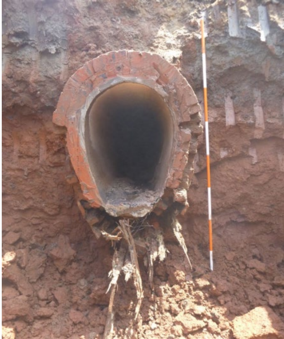
Figure 89. Cross-section of the Trumbull Street sewer, with wooden planks in the invert. Source: Ilene Grossman-Bailey and Laura D. Cushman, Trumbull Street Flood Control Project, Trumbull Street, East Sixth, Street and Bond Street, Block 7, Lot 1227, City of Elizabeth, Union County, New Jersey (Cranbury, New Jersey: Richard Grubb & Associates, Inc., 2019), 2-21.
