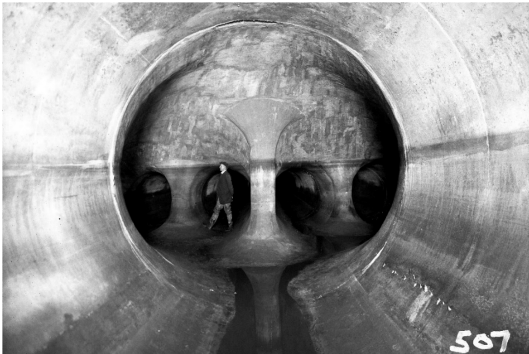
Figure 6. Passaic Valley Sewerage Commission interceptor. Source: Passaic Valley Sewerage Commission, Construction of Interceptors, for PVSC, 1920s. https://www.nj.gov/pvsc/who/history/photos/images/plant/img023.jpg
