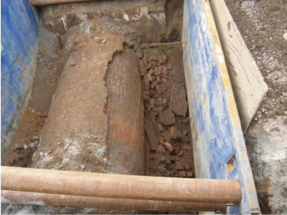
Figure 86. Exterior of the Arch Street brick sewer. Source: Robert J. Lore and Michael Tomkins, Archaeological Monitoring CSO Solids/Floatables Control Facility 005 Brick Sewer Documentation City of Paterson, Passaic County, New Jersey (Cranbury, New Jersey: Richard Grubb & Associates, Inc., 2008), 18.
