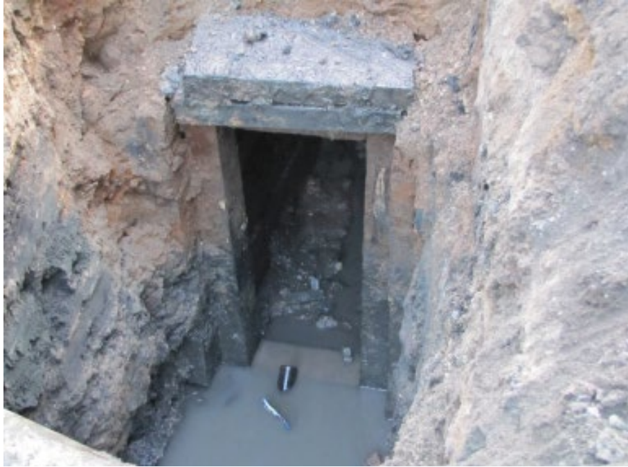
Figure 64. Photograph of the exterior of the Grand Street wood sewer. Source: Laura Cushman, Michael Tompkins, Amy Raes, and Paul McEachen, Archaeological Monitoring, North Hudson Sewerage Authority, Grand Street Combined Sewer Rehabilitation, City of Hoboken, Hudson County, New Jersey (Cranbury, New Jersey: Richard Grubb & Associates, 2015), 4-17.
