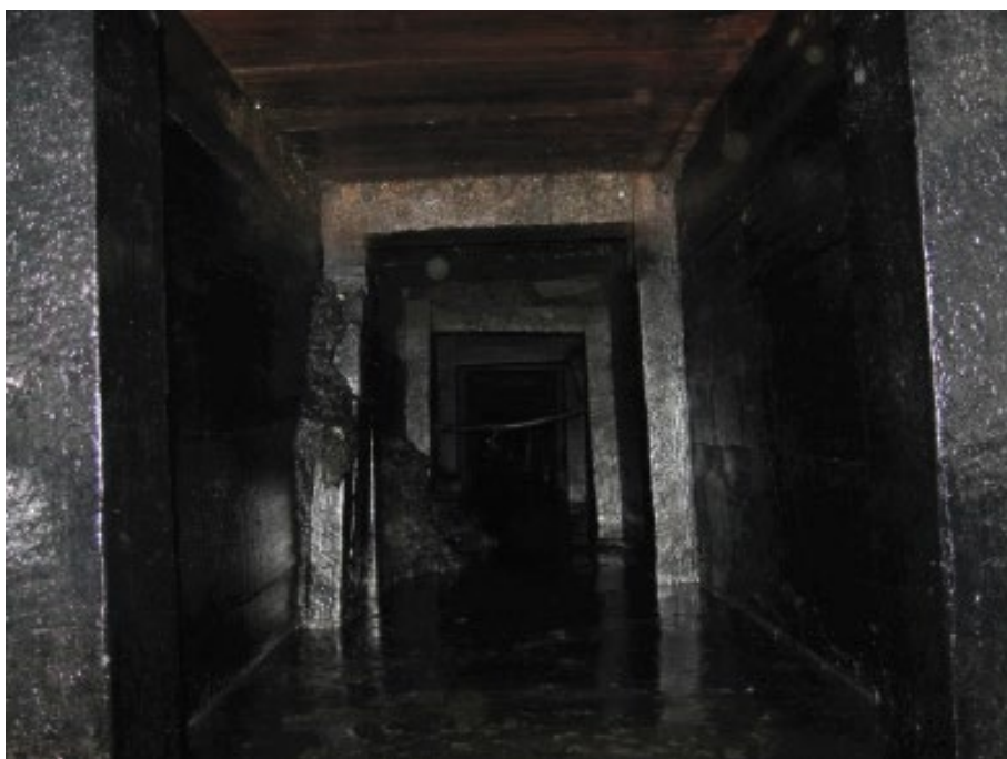
Figure 63. Photograph of the interior of the Grand Street wood sewer. Source: Laura Cushman, Michael Tompkins, Amy Raes, and Paul McEachen, Archaeological Monitoring, North Hudson Sewerage Authority, Grand Street Combined Sewer Rehabilitation, City of Hoboken, Hudson County, New Jersey (Cranbury, New Jersey: Richard Grubb & Associates, 2015), Appendix E.
