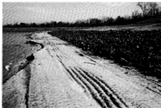
The installation of riprap on the saddle area between the dam and the dike at the Manasquan Reservoir in Howell Township.
