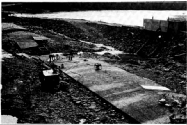
Rehabilitation of the Lumberville Wing Dam spanning the Delaware River between Delaware Township, NJ and Plumstead Township, PA.
