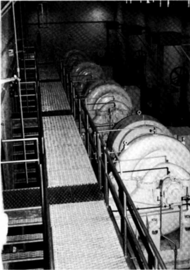
Four of the ten 2,000 HP pumps located at the South Branch Pumping Station used to pump water into the Round Valley Reservoir.
