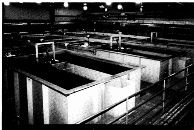
The three Filter Clarifier Units in the Water Treatment Plant have been rehabilitated.
