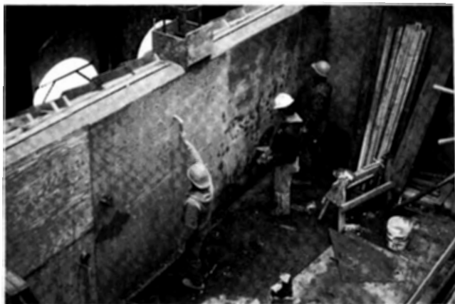
Completion of modifications to the Whitehouse Station Release Building in connection with the reduced pressure operation of the Round Valley Reservoir Release Pipeline.
