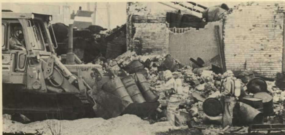
Workers in protective clothing remove burnt out drums from Chemical Control after the April 21 fire.
