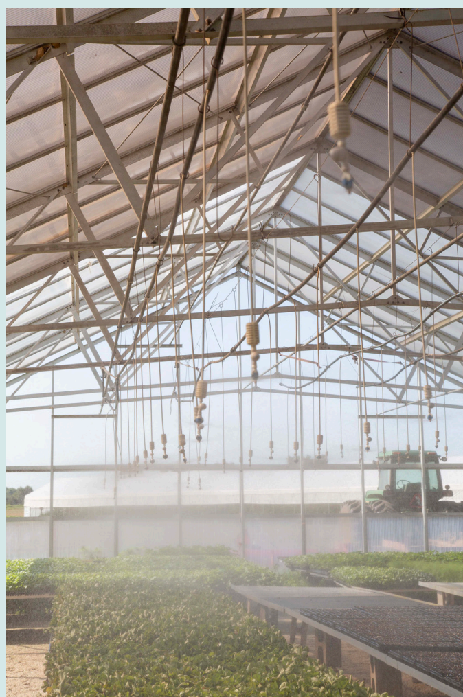
An indoor spray irrigation system located at Specca Farm in Bordentown, New Jersey.
