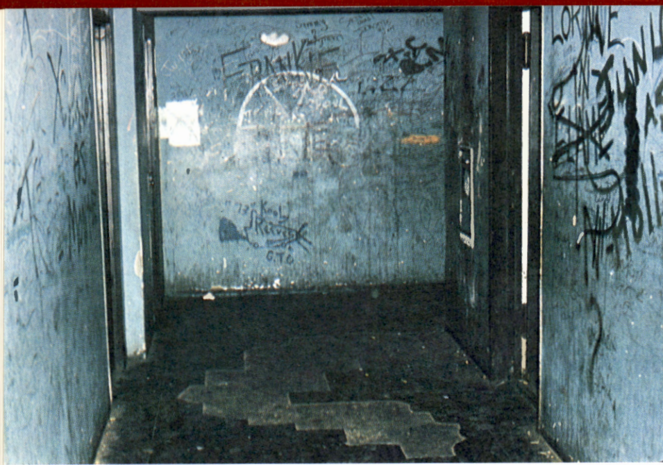
The condition of public hallways throughout A. Harry Moore epitomized the acute degree of resident frustration and hapless housing authority management in the early '70s. (A typical example, 1973.)
