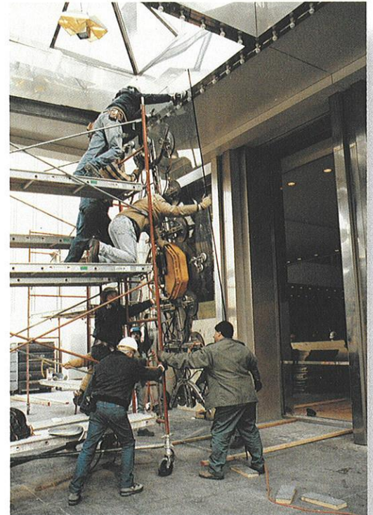
The monumental task of World Trade Center recovery was at the forefront of Port Authority attention in 1993.
