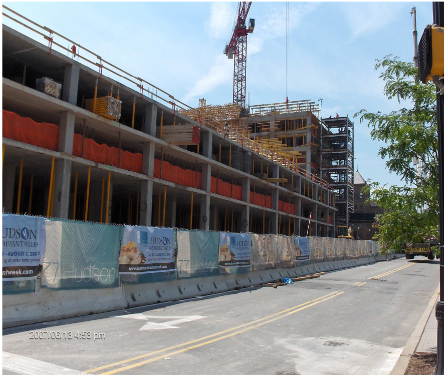
Work at the condominium development, 77 Hudson St., Jersey City. Photo by Drake Rizzo and Charles Pierson, Jr.
