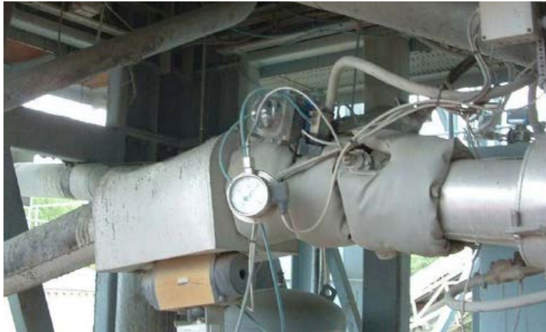
Figure 7. WAM Foam Expansion Chamber, Controls and Transfer Pipe
