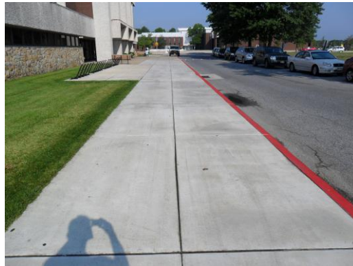
Figure 11. Condition of sidewalk in front of Robinson Hall on August 9, 2012
