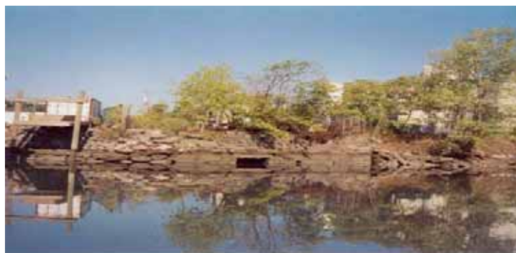
PURDY AVENUE (VILLAGE OF PORT CHESTER, NY) OUTFALL TO THE BYRAM RIVER (FACING WEST)
