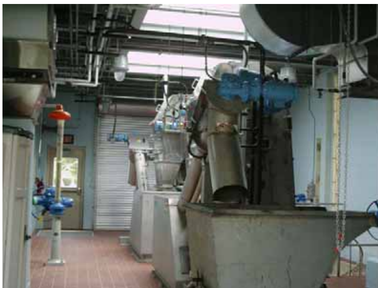
FINE SCREENS AND SCREENING INSIDE RENOVATED AND EXPANDED BUILDING
