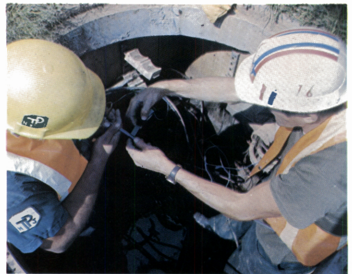
Repairing underground cables at a junction area—one of the myriad tasks of Maintenance.
