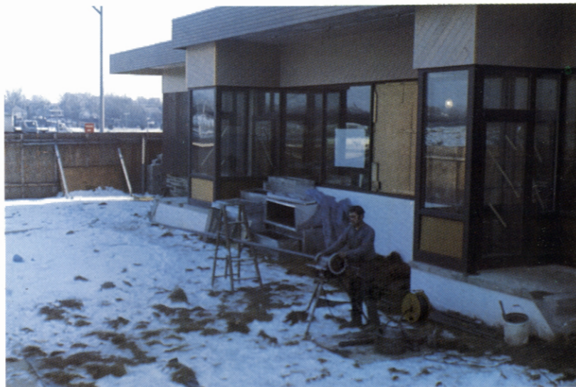
Undeterred by the weather, renovation goes on at Thomas Edison Service Area at Woodbridge.
