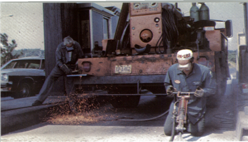
Here a Maintenance crew works on a lane treadle conversion at an interchange.
