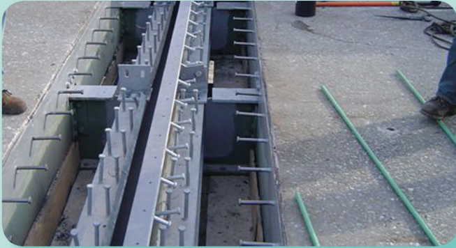
Some of the annual maintenance work on the DMB scheduled for this fall includes replacing expansion joints like those shown above and redecking the roadway where needed.
