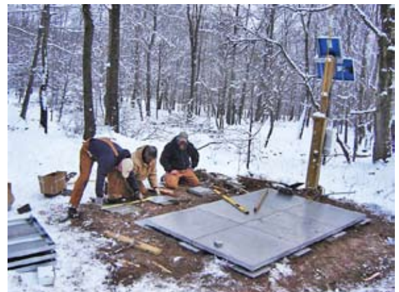
Members of the NYCDEP Watershed Monitoring and Operations Support staff install the first automated snowpack water equivalent monitor (or "snow pillow") in the Neversink Watershed in January 2008. (Photo courtesy of NYCDEP)
