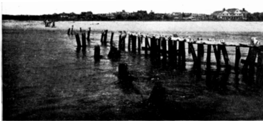
Fig. 1. Looking Across the Inlet, September, 1915, to the Avon Shore. Remains of the Concrete Piling Undermined by the Current; Old Wooden Jetty at Right.
