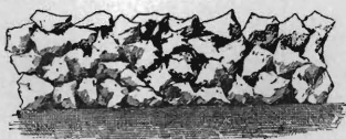
Stone on a macadam road as it appears when spread ready for rolling.
