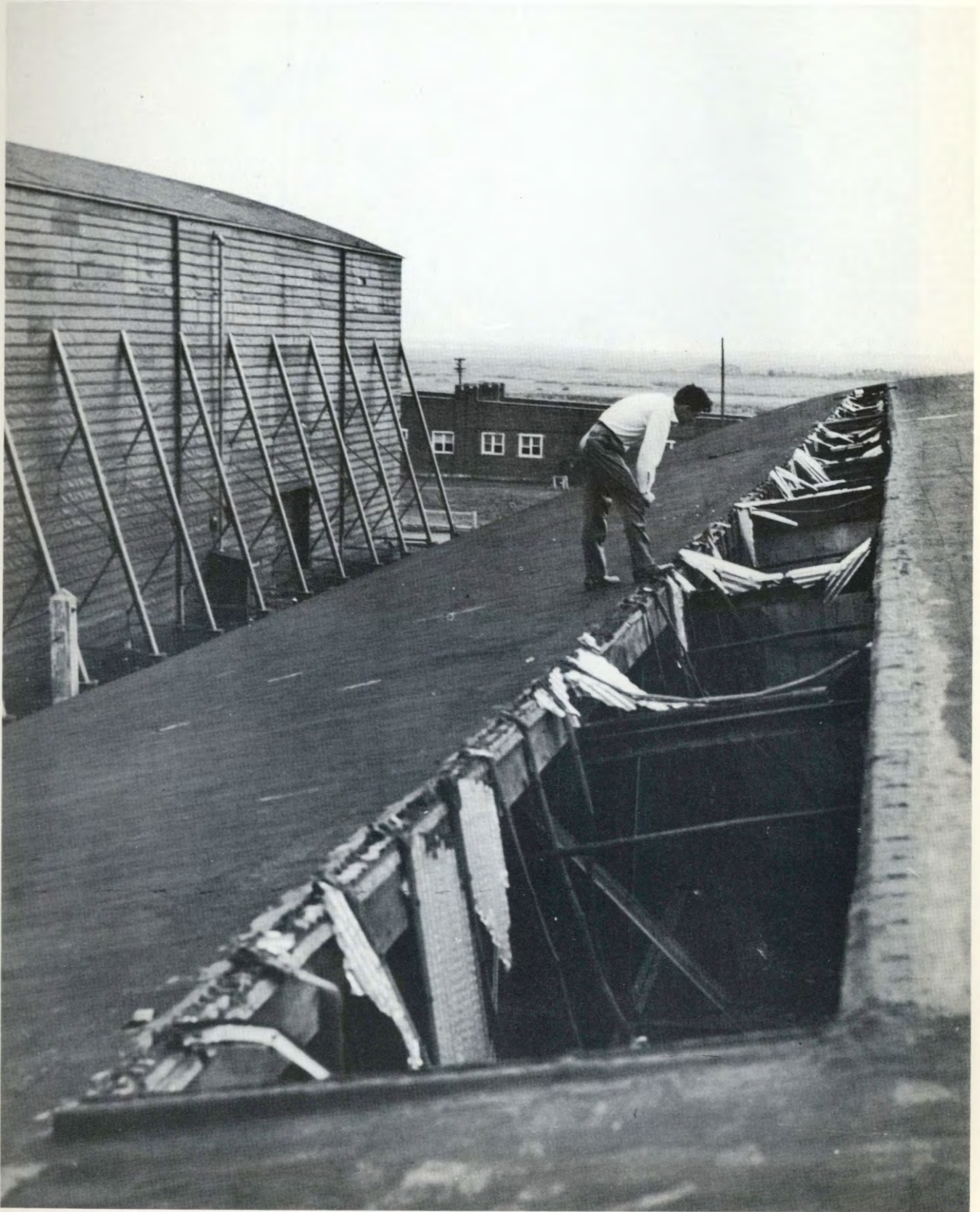
BUILDING 103, SEARS-ROEBUCK AREA, SHOWING BROKEN SKYLIGHTS.
