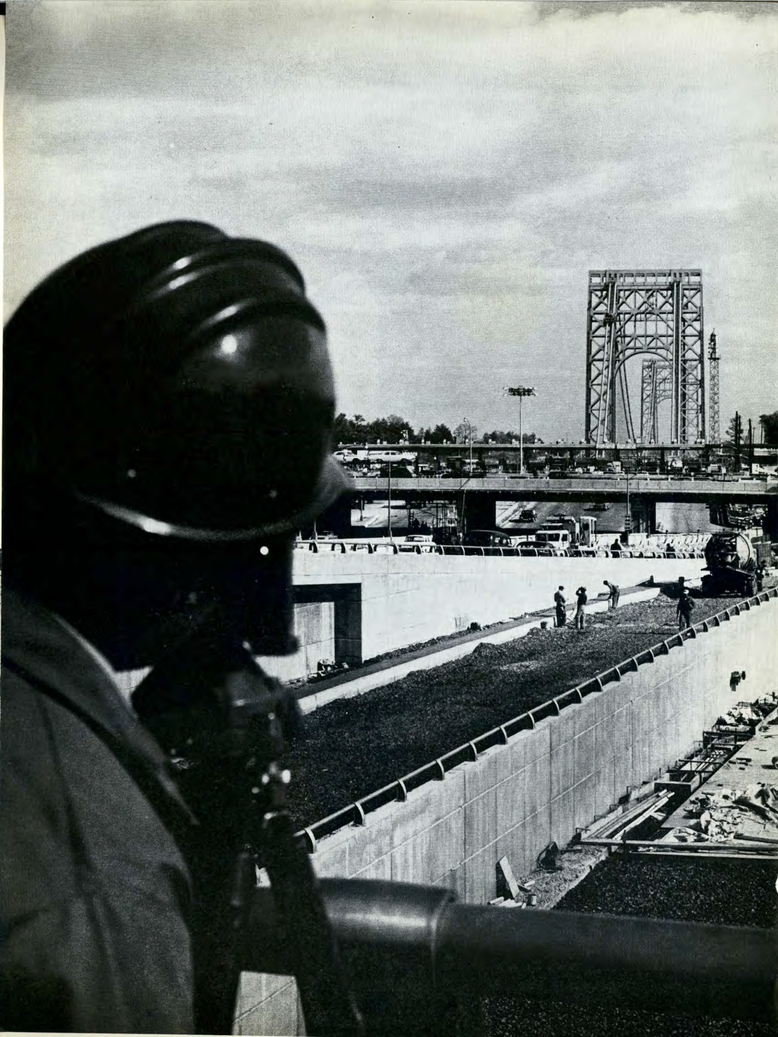
Traffic flows steadily on the New Jersey approaches to the George Washington Bridge during intensive construction activity on the lower level project.
