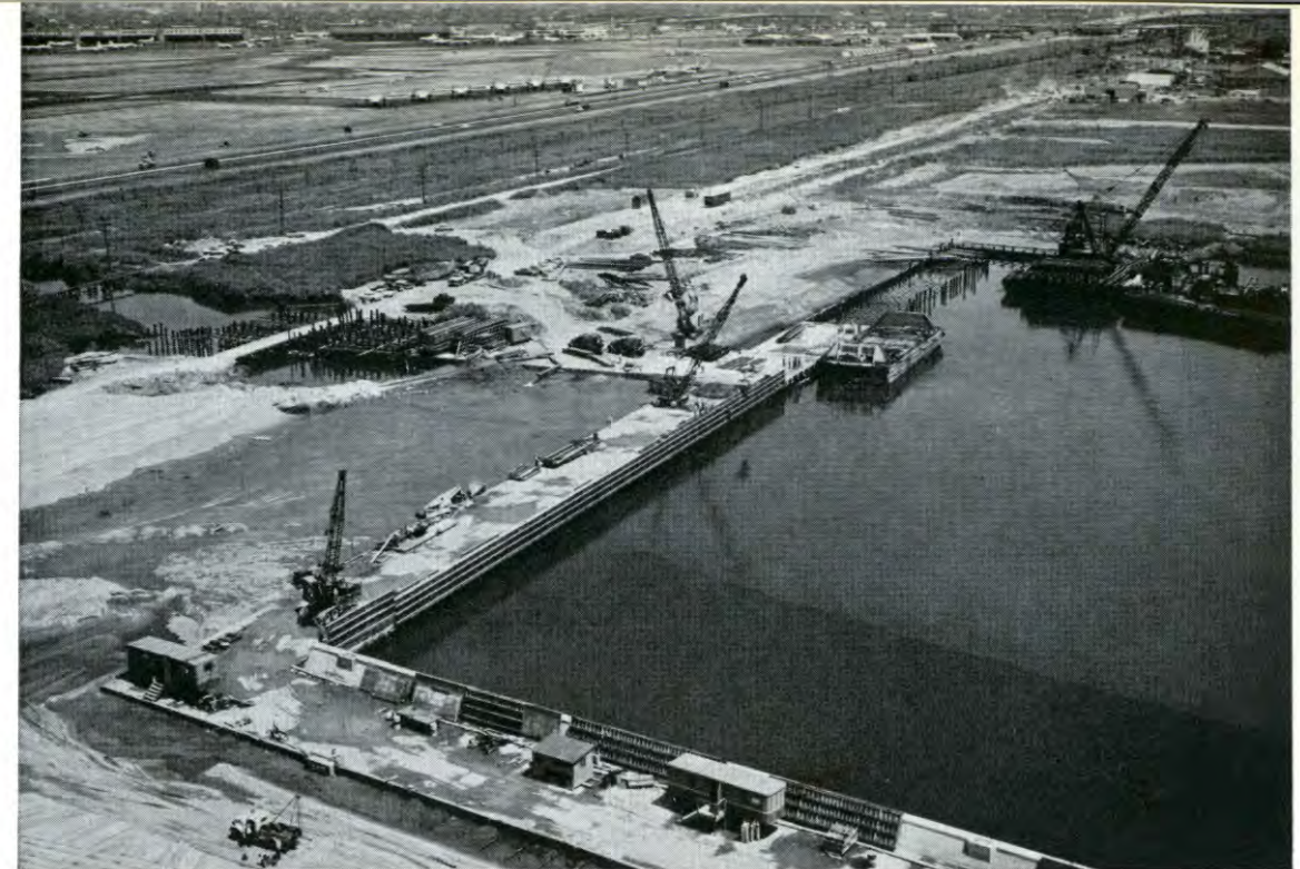
Development of the Elizabeth-Port Authority Piers progressed rapidly in 1961 with construction of wharves, aprons, and distribution buildings. The photograph shows work underway at the head of the 9,000 ft. Elizabeth Channel.
