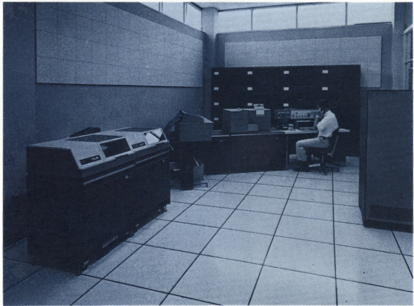
Container Control Center
