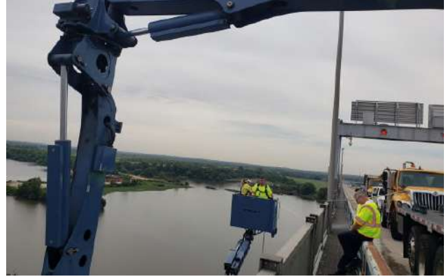
Ongoing maintenance includes pressure washing various sections of bridges to combat corrosion.
