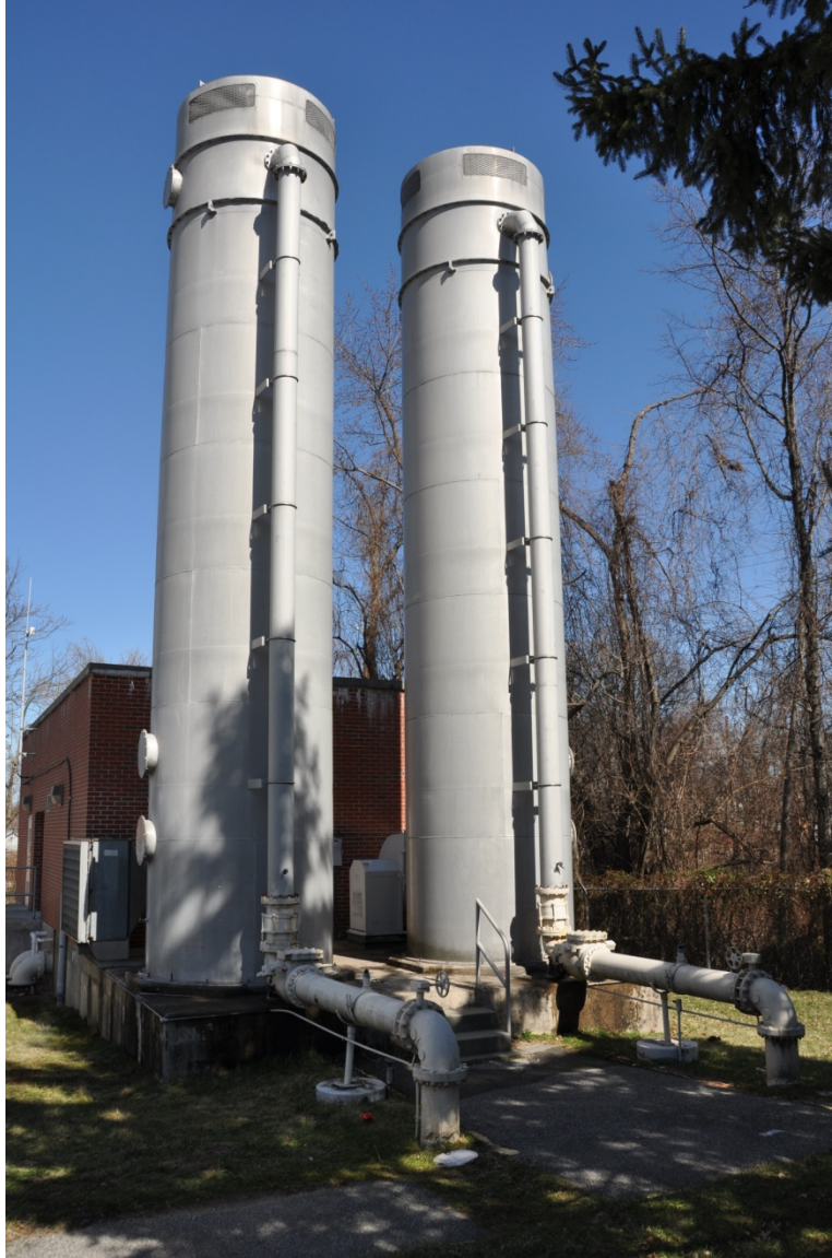
Figure 1. Supply wells and air stripping units at the Merchantville/Pennsauken Marion Avenue facility.
