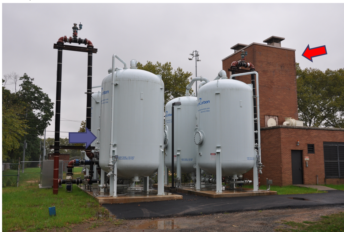
Figure 4: Depiction of the Fair Lawn Cadmus Avenue Facility GAC Contactors. The red arrow on the right identifies the air stripping unit present at the facility and blue arrow highlights the location of the sampling ports for the four different bed depths.
