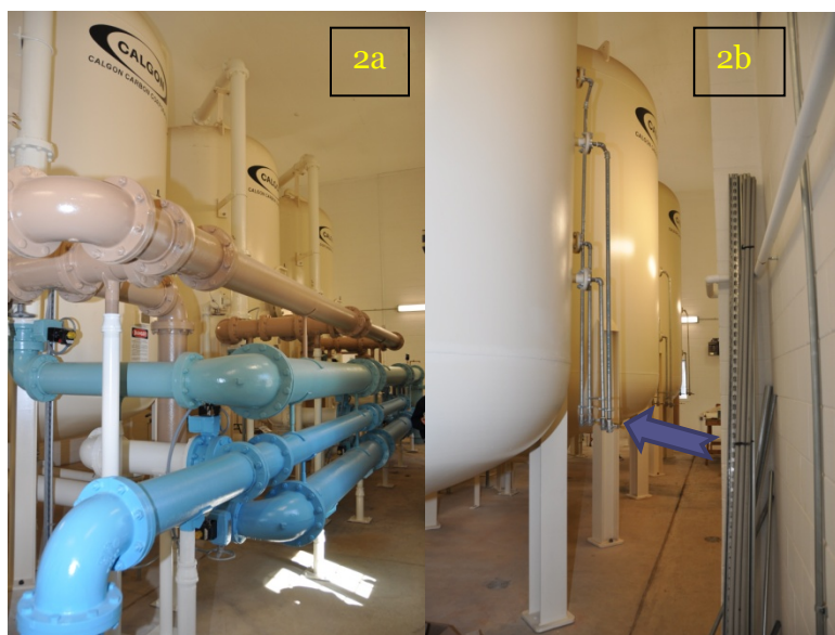
Figure 2a and 2b. Depiction of the front (a) and back (b) of the GAC pressure vessels configuration at the Merchantville/Pennsauken Marion Avenue Facility. The arrow in 2b shows the location of the four pressure vessel depth sample taps.
