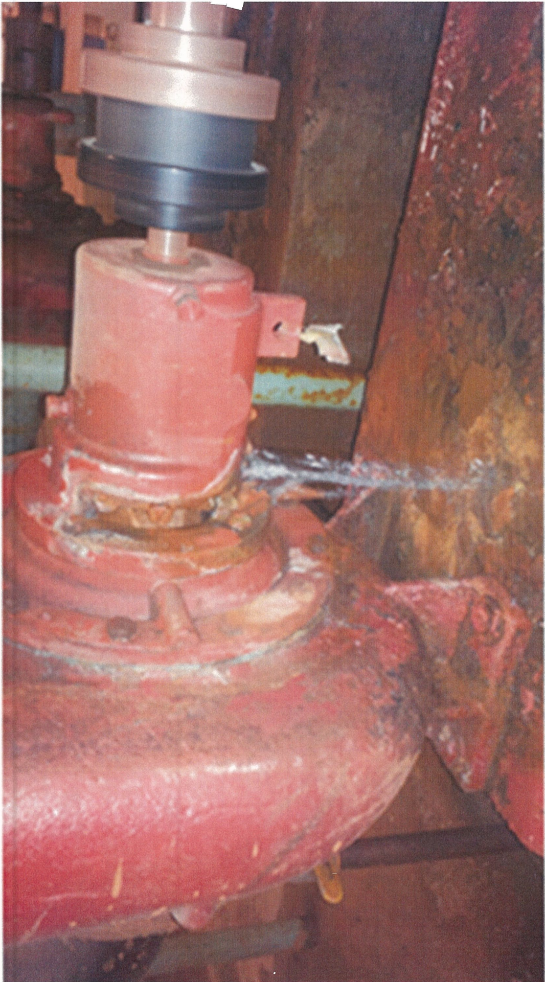
OHS Leaking Water Pump
